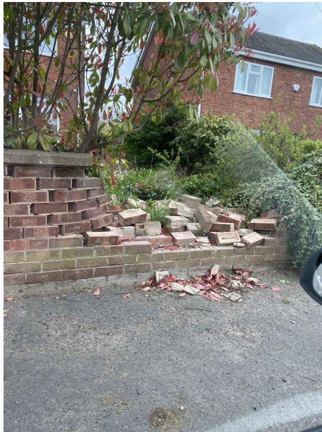
Figure 6: Collapsed wall in South Kelsey. Image: Logan Roe
